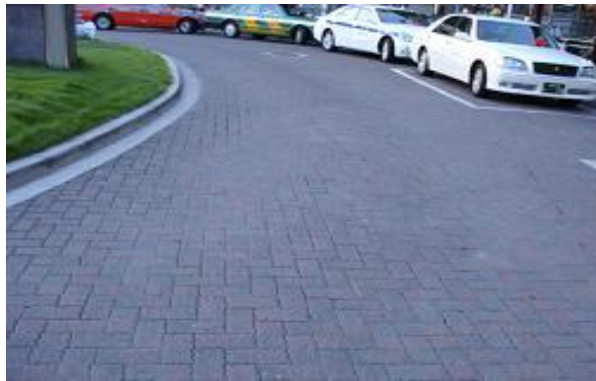
Figure 4. Rutting near taxi bay.
