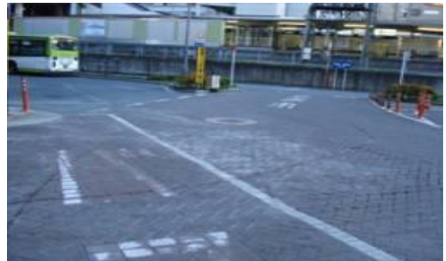
Figure 5. Damaged area at part of bus station.
